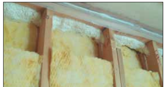
Construction monitoring verifies that a gap between party walls has been sealed air tight with closed cell foam.
